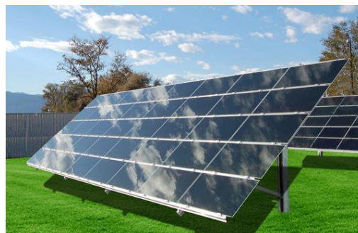
A Typical thin film photovoltaic array
